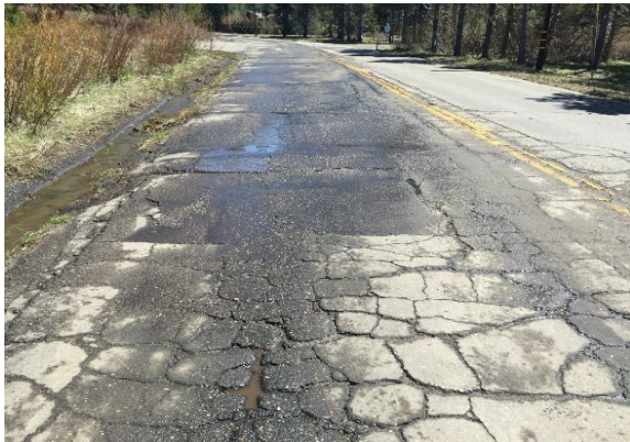
Figure 73 Elks Club Drive in 2018 prior to repaving. (R Wigart)
