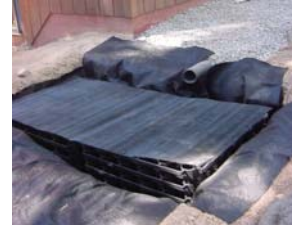
Rainstore with Geotextile
