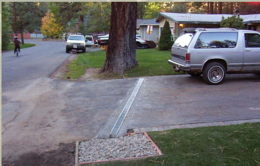
Slotted channel drains convey driveway runoff to drain rock infiltration systems or drywells.
